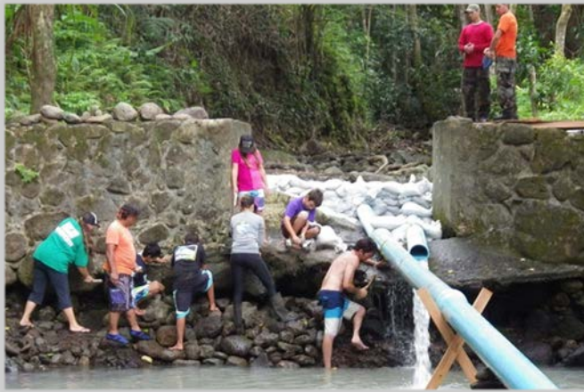
Volunteers, and partners prepare the Waihee site for construction. Credit: Gordon Smith/USFWS
