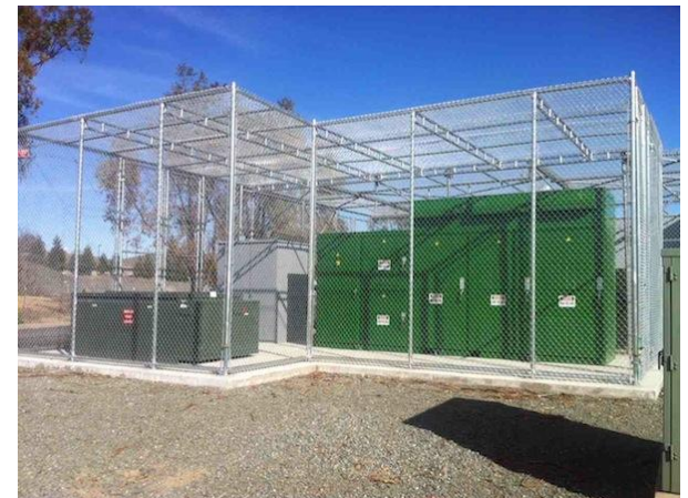
PCC Controls at Santa Rita Jail
