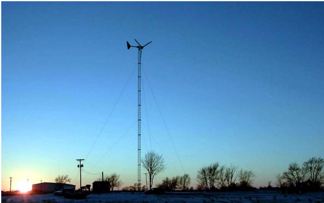
Groundwater recirculation well powered by a wind turbine at the Former Nebraska Ordnance Plant Superfund Site, Mead, NE. Photo by Ernie Guitierrez and used with permission of Curt Elmore, Missouri University of Science and Technology
