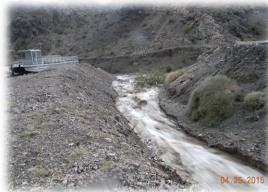
Water Flowing Below the Gabion Structure
