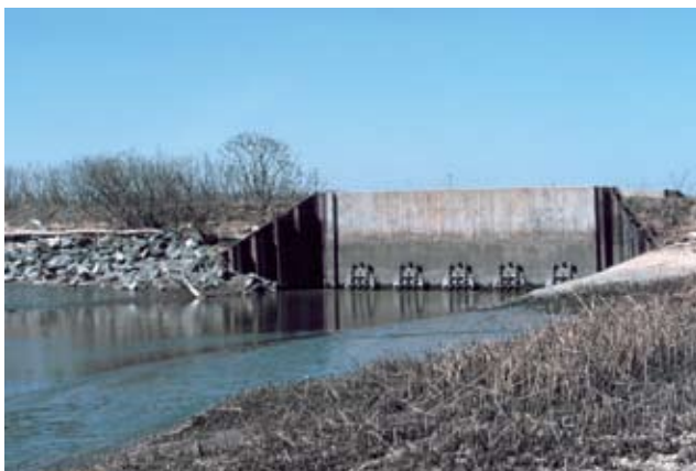
Figure 6.5 The tide gate at the mouth of Army Creek on the Delaware side of the Delaware River. The tide gate drains flood and rain water out of the creek to prevent flooding. The five circular mechanisms on the gate open and close to control water flow [Photo source: courtesy NOAA Photo Library].
