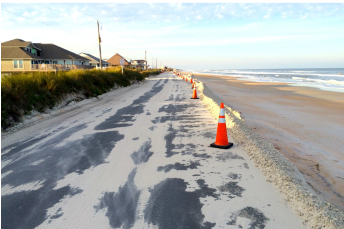
Figure 80. Erosion along Old A1A
