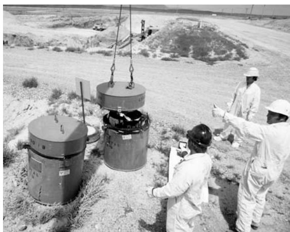
Waste Receiving and Processing at Hanford Site.
