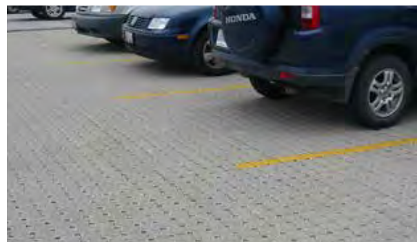
Open joint pavers provide opportunity to retain rainwater and snowmelt on-site
