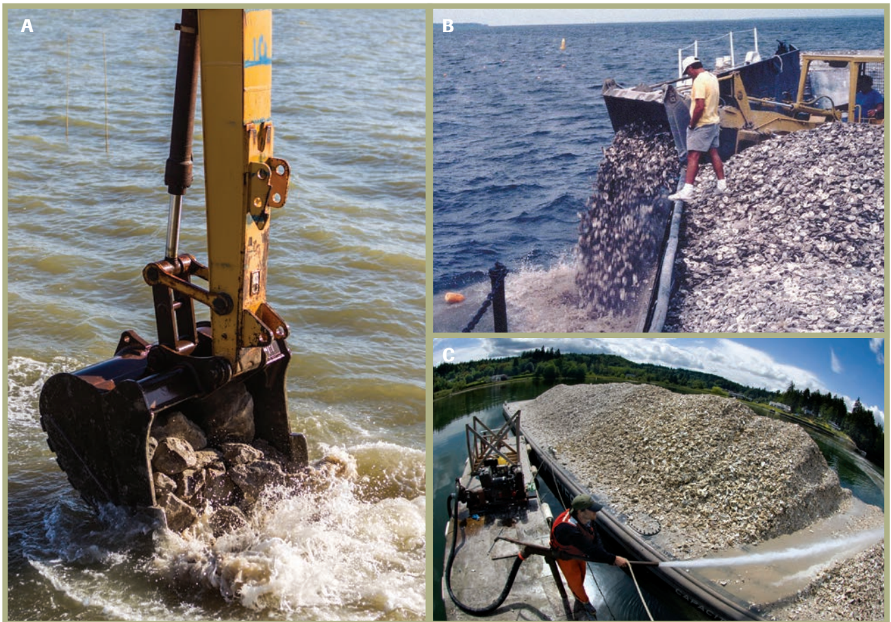
Figure 5A, B and C. (A) Limestone marl being placed as reef substrate in Matagorda Bay, Texas. (B) NC DMF vessel delivering marl to restoration sites. (C) Using a water cannon to spread oyster cultch over a restoration site in Dogfish Bay, WA.
