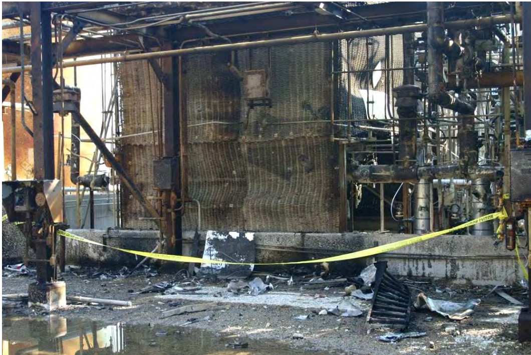
Figure C-1. MIC tank blast shield post-incident
