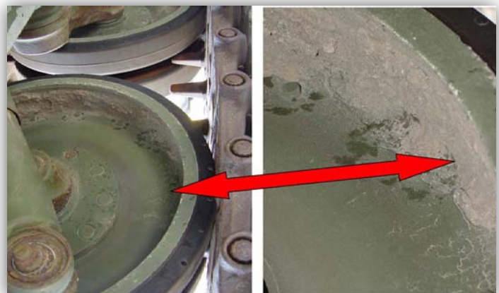
Right: Inner view of track roller. Post-inspection on a previously cleaned vehicle, note the remaining mud accumulation. This photo illustrates the value of an equipment inspection following cleaning (Photo credit: Bureau of Reclamation).
