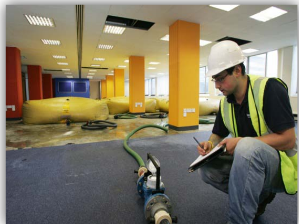
Crane testing companies often provide certification that the water bag was filled only with potable water at its last location, or was filled with raw water and properly decontaminated. If there is any doubt, insist upon decontamination of the water bag before allowing its use at the facility (Photo credit, Imes, Inc).
