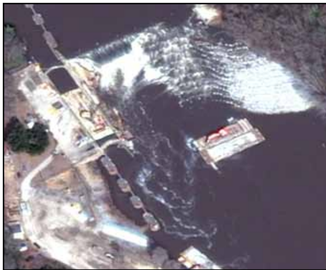
Aerial view of the rock arch ramp fishway under construction at Lock & Dam #1.
