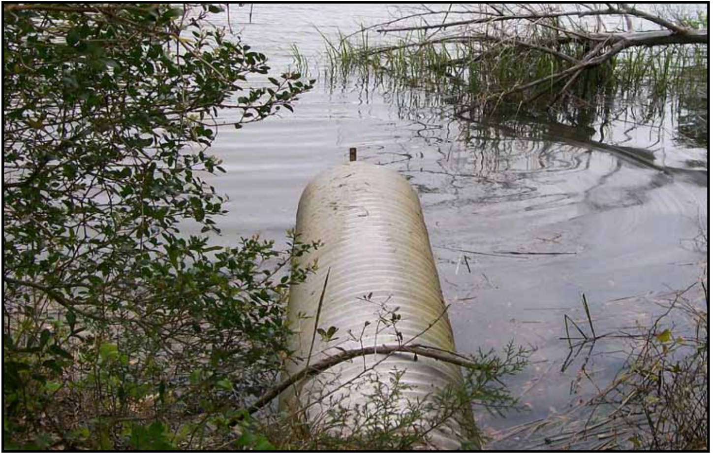
Stormwater pipe. Photo courtesy of NCDWQ.
