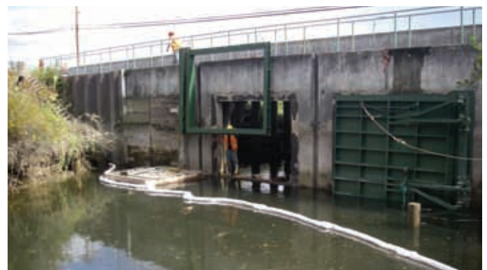
New floodgates installed on Fisher Slough in Washington's Skagit Delta. ©Jenny Baker/TNC
