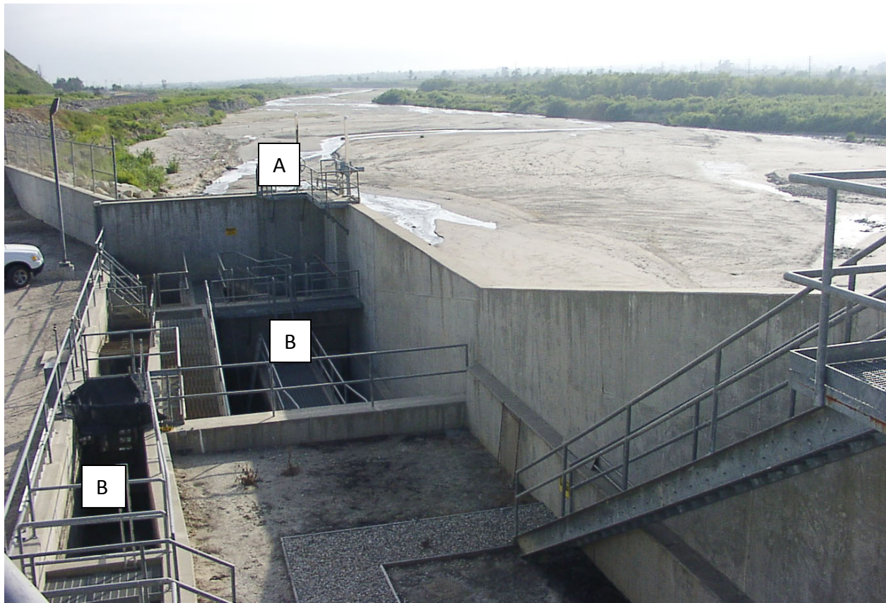
Figure 14. Vern Freeman Diversion Denil fish ladder, looking downstream, Santa Clara River. A - Fish ladder entrance. B - Denil fish ladder segments.
