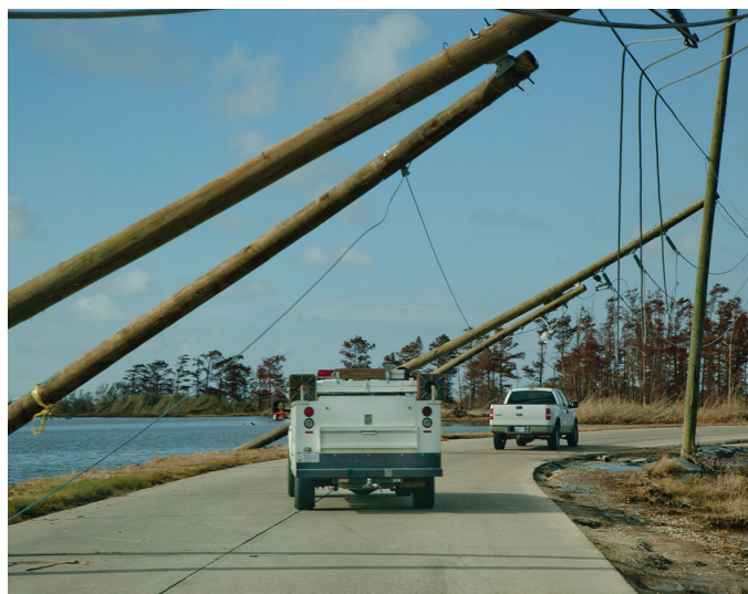
Power lines damaged by Hurricane Isaac's wind and surge in Plaquemines Parish, Louisiana, September 3, 2012.
