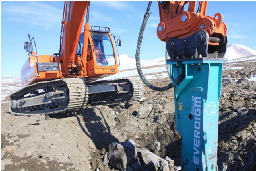
Digging through continuous permafrost to install towers that were part of the new isospheric research radar in Antarctica. Justin Mabie/CIRES
