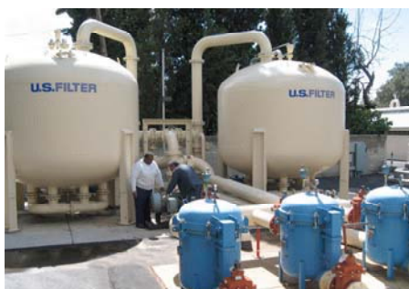
Technicians conduct maintenance at the NASA-funded Lincoln Avenue Water Company groundwater treatment plant. Shown above is the ion exchange system that removes perchlorate from water. Another section of the plant, not shown, removes volatile organic compounds from the water.
