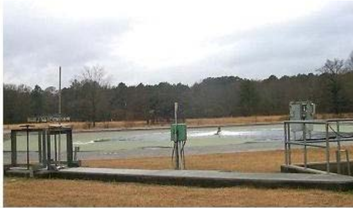
Yemassee waste water treatment plant
