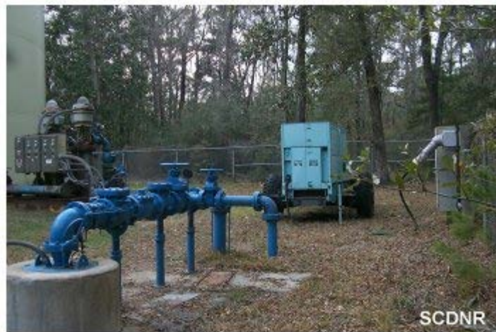
Edisto Beach public works well head
