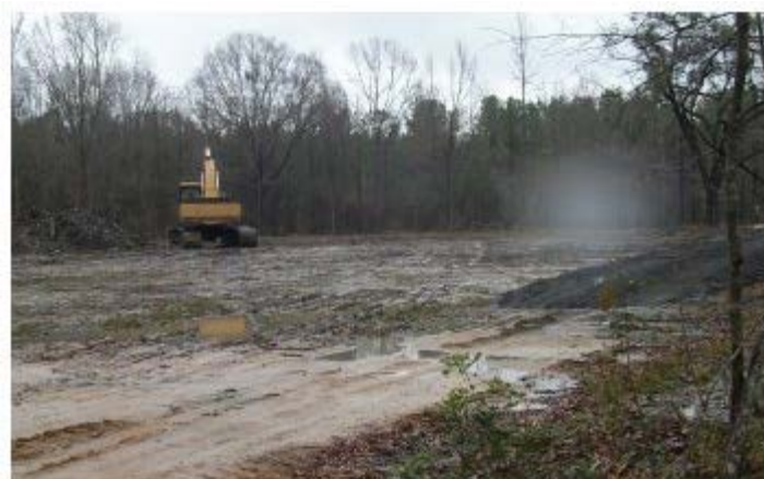
Runoff from cleared construction site
