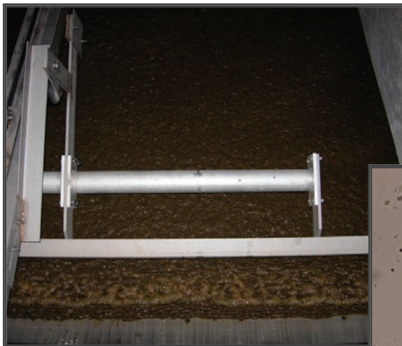
Algae skimmer removes biomass in a dissolved air flotation plant in Waco, Texas
