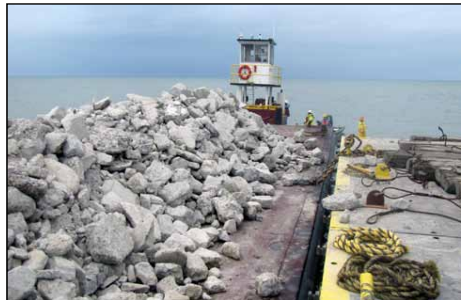
Reef material is staged at the jobsite in preparation for the construction of the $1.3 million Half Moon Reef project to restore 12 acres of sub-tidal reef and habitat located within the northernmost extent of the Half Moon Reef in Matagorda Bay, Texas – one of the largest restoration projects around the country.
