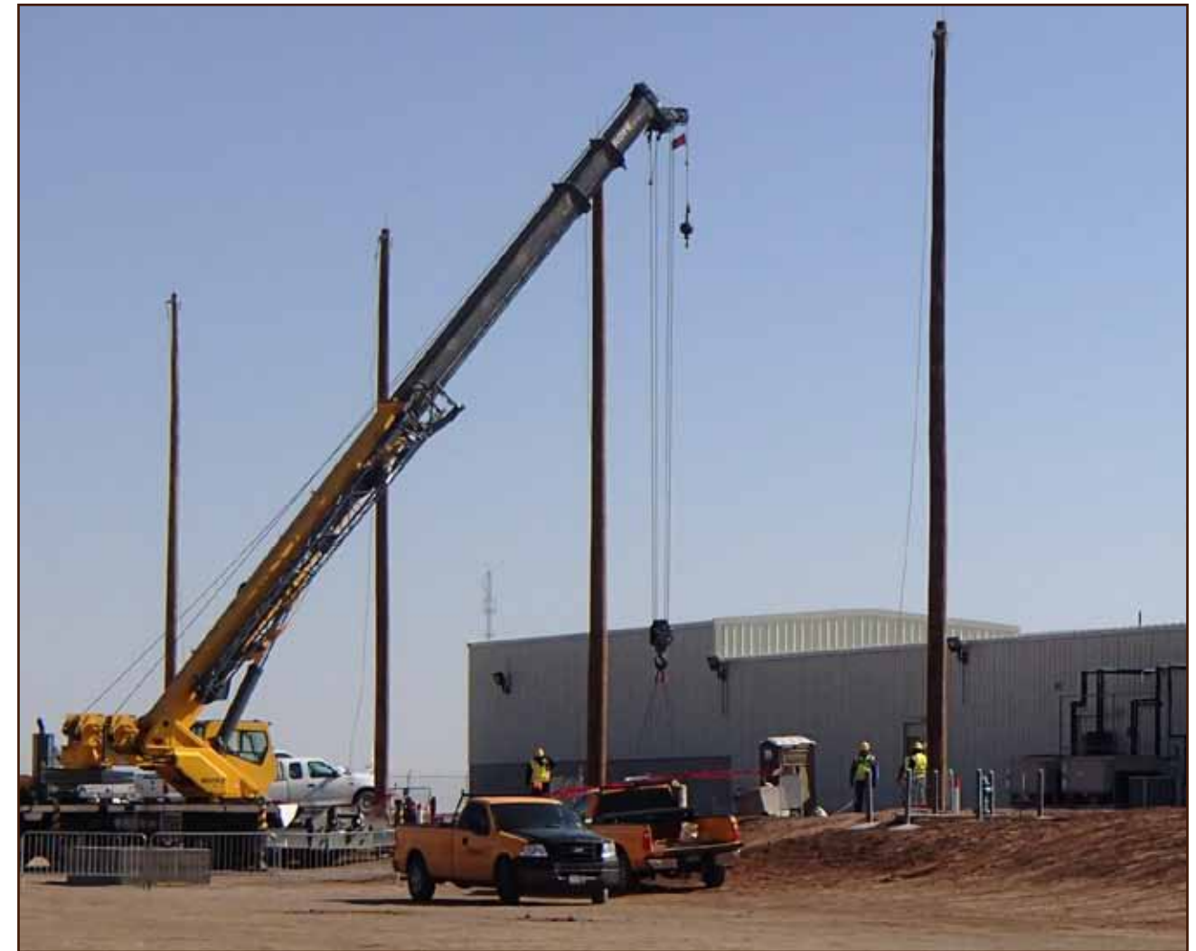
Crews are putting the final touches to the High Explosive Production Facility complex on Department of Energy's plant near Amarillo. The project is expected to provide a consolidation of several buildings on the plant grounds for higher efficiency and safety. (Photo courtesy of Sydney Brainard)
