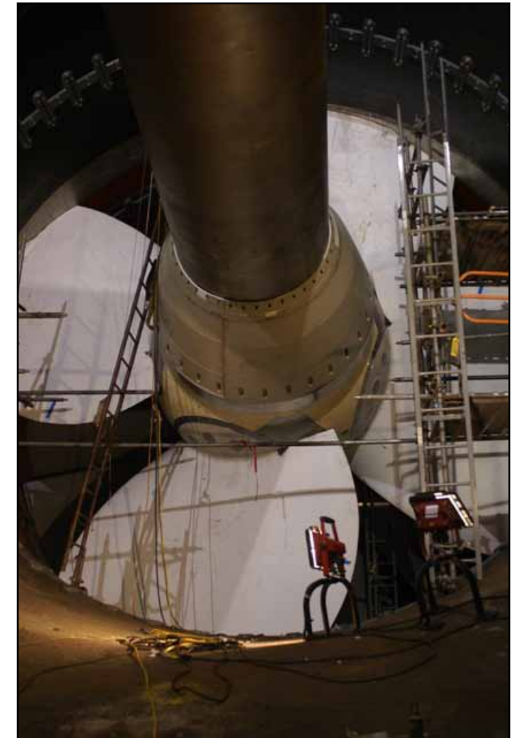
The second of three turbines have been installed at Webbers Falls as part of a major rehabilitation effort sponsored by Southwestern Power Administration and funded through customer fees. (Photo by Brannen Parrish)
