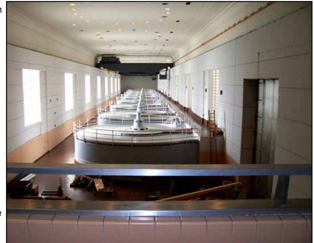
Bull Shoals Powerhouse is one of seven hydroelectric generating plants in the Little Rock District that receives capital improvement funds through a cost sharing agreement with Southwestern Power Administration and the Southwest Preference Customer Trust. (Photo by Little Rock District)
