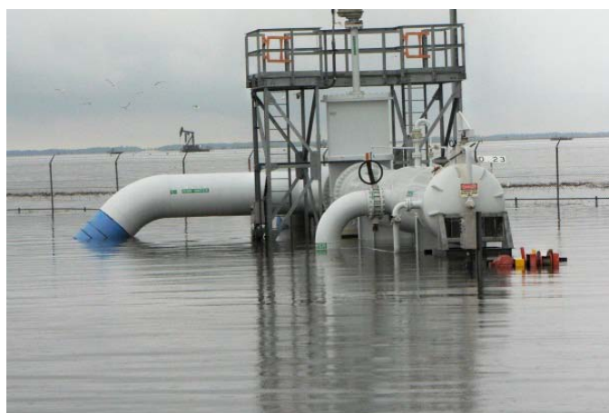
Figure 23. SPR site and equipment inundated following a storm surge
