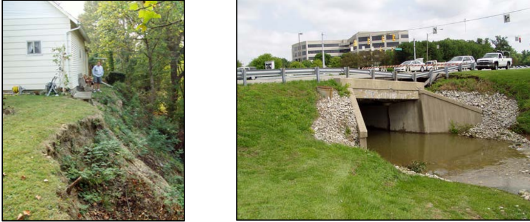
Figure 6. Examples of impacts of fluvial-erosion hazards in Indiana include the threat of loss or major damage to a residence (left) and damage to a heavily travelled urban bridge in Indianapolis (right).
