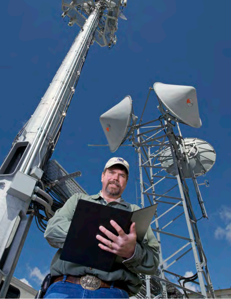
Worker monitoring communication towers within CITRC.
