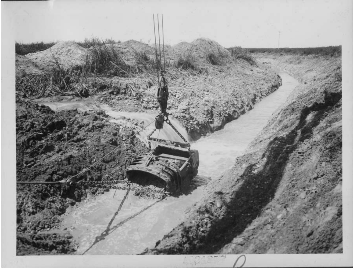
Figure 23 June 22, 1914 "Dredge bucket loading in hard cemented gravel on Purdam Slough Drain." 109
