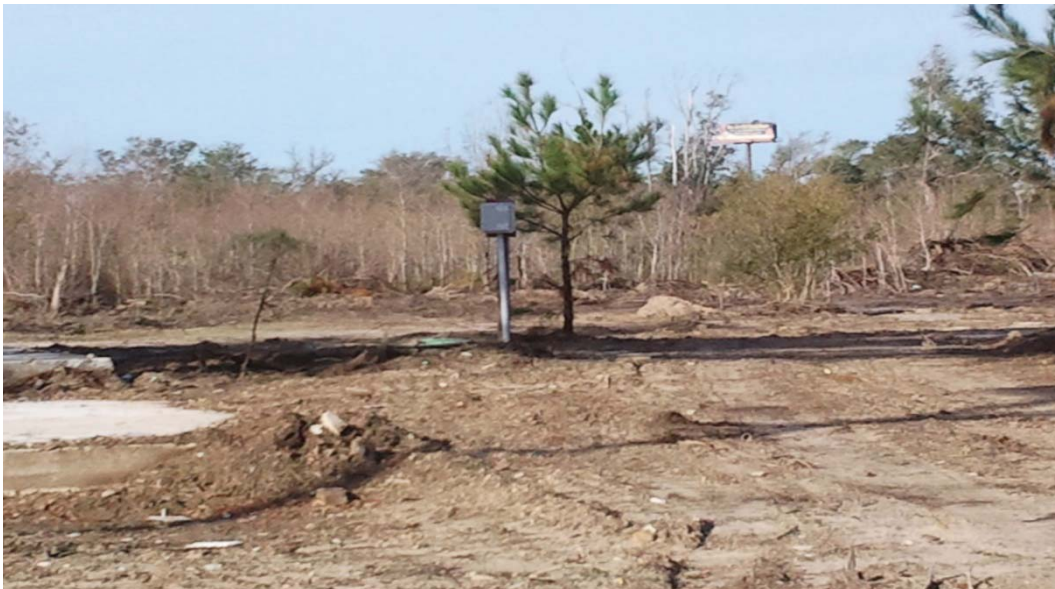
Figure 3: Grinder pump and control panel located at 150 Lady Mary in Henderson Point. The grinder pump is not currently attached to a residence. Source: OIG site visit (December 28, 2011).
