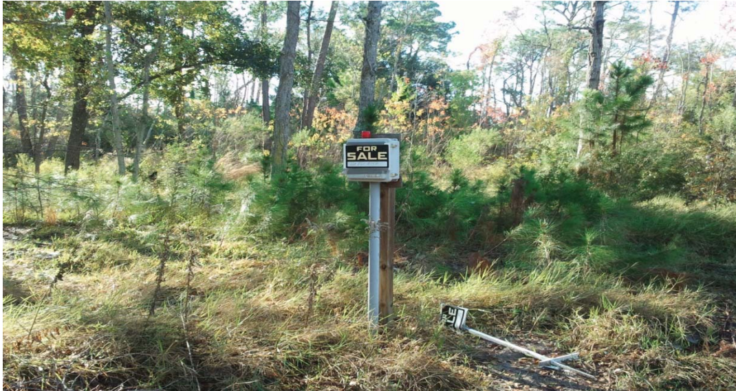
Figure 2: Grinder pump and control panel located at 300 Audubon Lane in Henderson Point. The grinder pump is not currently attached to a residence. Source: OIG site visit (December 8, 2011).
