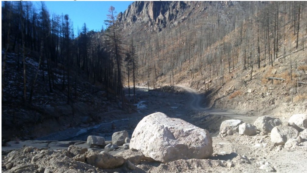
Figure 1. Damage to Santa Clara Canyon Road after repeated disasters.
