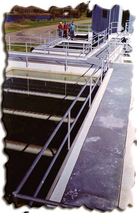
Planning Assistance to States (PAS) includes performance evaluations of water treatment plants.
