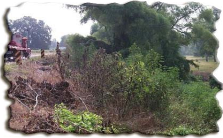
The banks of a bayou are overgrown and flood waters are slowly eroding the bank and endangering the highway.
