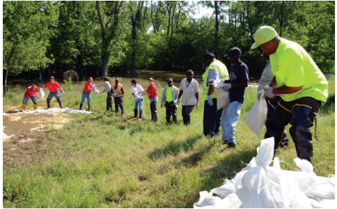
Workers place sandbags near a developing sand boil during the high water event of 2011.
