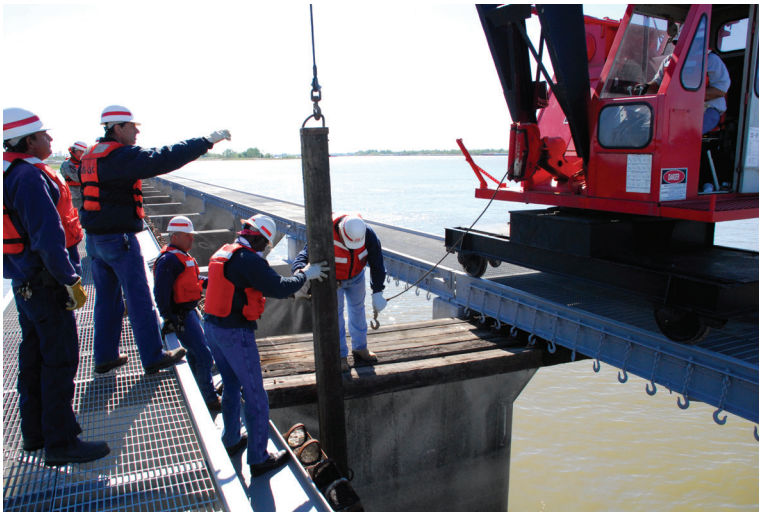
In opening the spillway, each timber is individually lifted and placed atop the structure.
