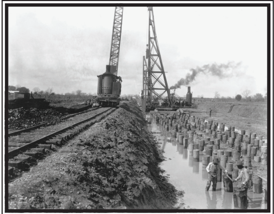
Thousands of wooden pilings were driven to provide a reliable foundation for the spillway structure.
