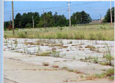
Fig 5.28 – Over abundance abandoned concrete foundations overgrown parking lots
