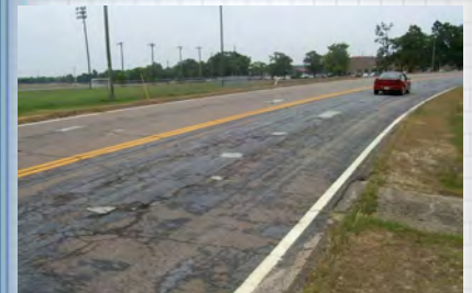
Fig 5.24 – Deteriorated road surfaces
