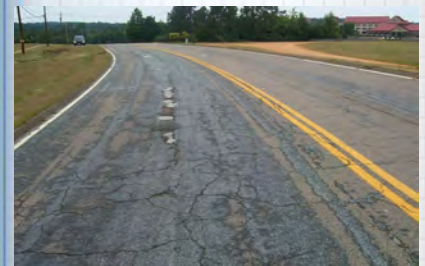
Fig 5.31 – Deteriorated road surfaces
