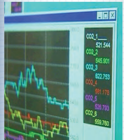
1.2 - CO2 Measurements Measure Indoor Air Quality Assisting in Creating a Healthy Environment
