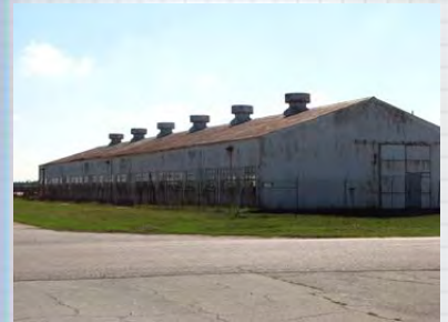
Fig 5.27 – Some older buildings in disrepair
