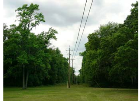
Fig. ES.78 - Routing transmission lines in wooded areas reduces their visibility.
