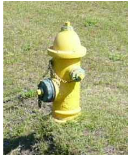
Fig. ES.79 - Fire hydrants are yellow with color-coded markings on the cap that indicate flow rate.
