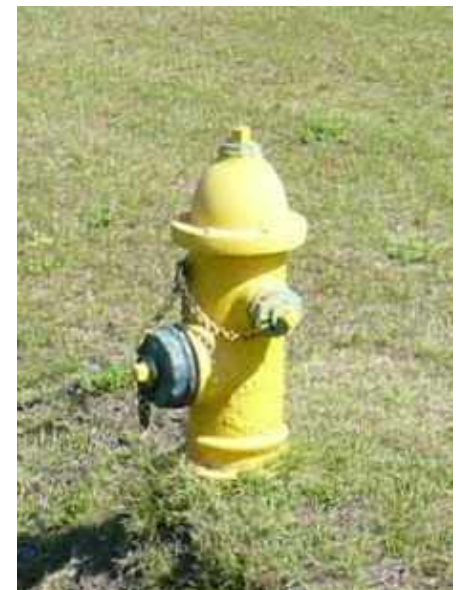
Fig. ES.80 - Fire hydrants are yellow with color-coded markings on the cap that indicate flow rate.
