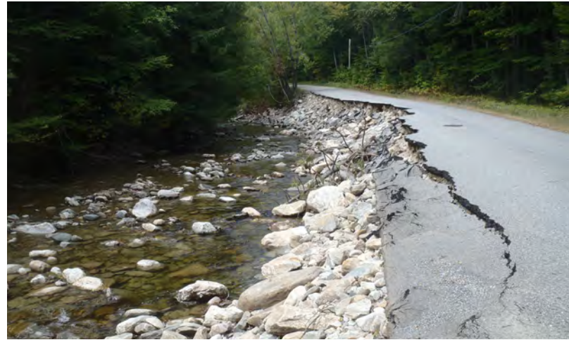
A stream channel erodes causing the bank and adjacent road surface to collapse.
