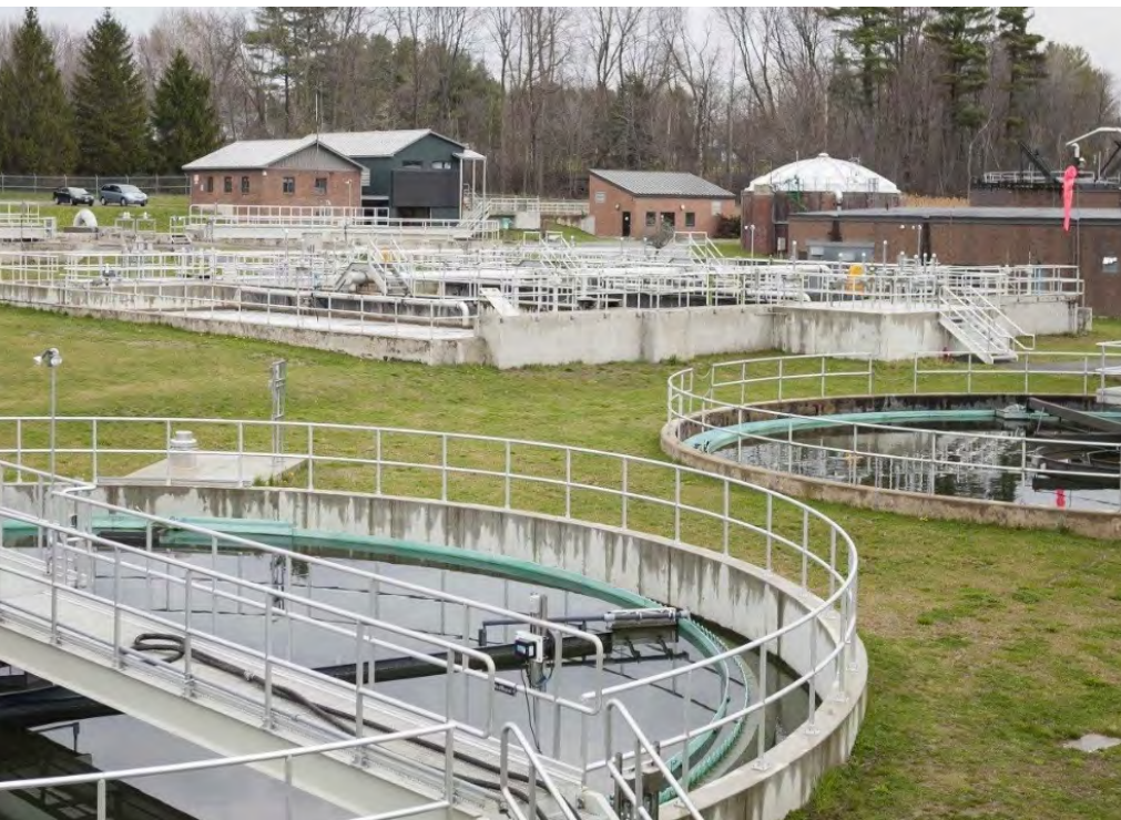
Wastewater treatment facility in Vermont.
