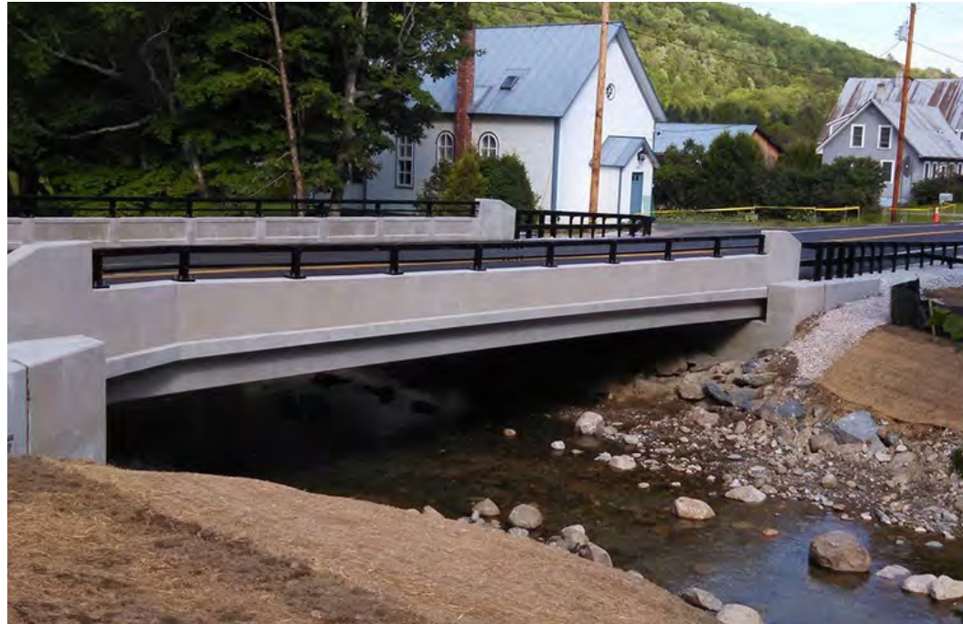
Erosion prevention and sediment control practices associated with a VTrans bridge-replacement project.
