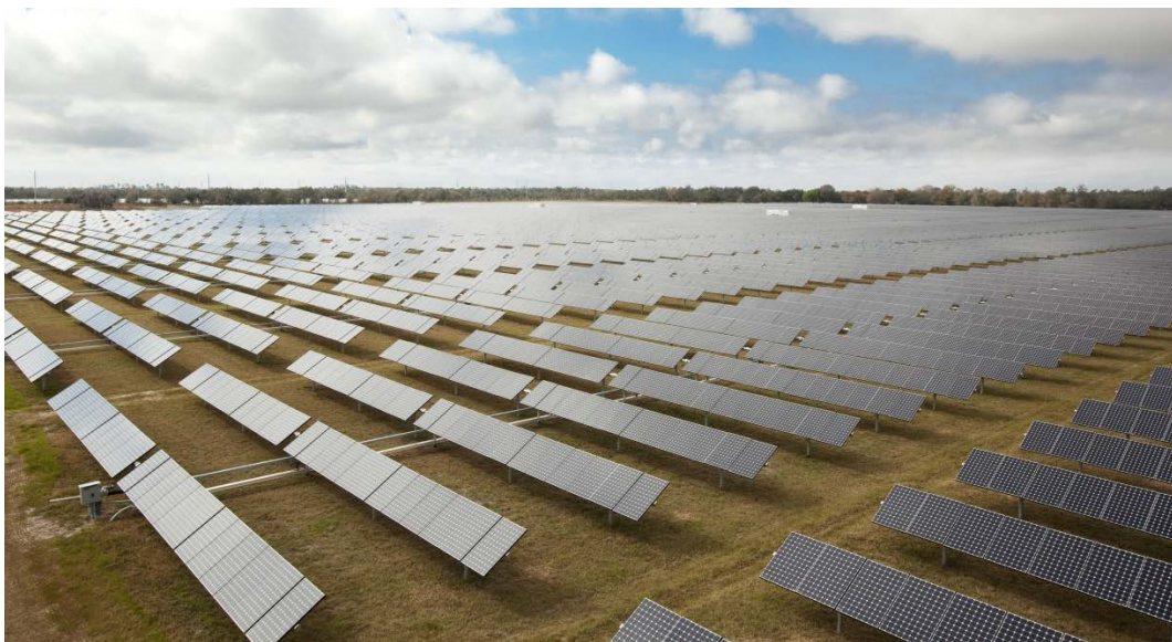
Figure A11. PV arrays placed in a fixed-tilt position or mounted on a tracker. Photo by NREL
