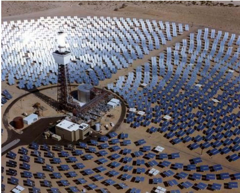
Figure A17. A molten-salt power tower. Photo from NREL
