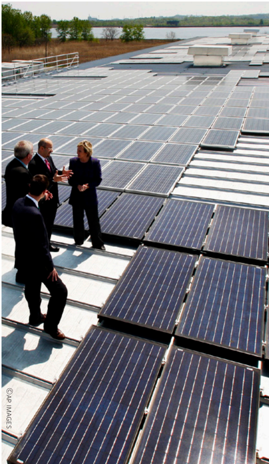
More than 12,000 solar panels cover 1.2 hectares of roof space on a Federal Express building in Woodbridge, New Jersey.
