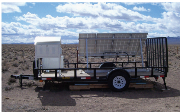
Station 401, Solar Powered Air Sampler
