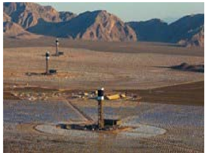
The Ivanpah Solar Energy Generating System, located in the Mojave Desert, is the largest solar thermal energy facility in the world. DOE provided a $1.6 billion loan guarantee to the project. (Photo courtesy of Gilles Mingasson/Getty Images for Bechtel)
