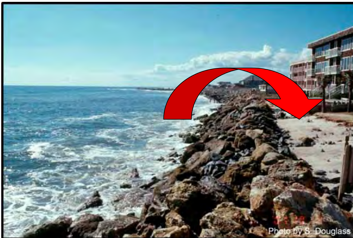
Figure 6.16. An example of splash damage behind seawall
