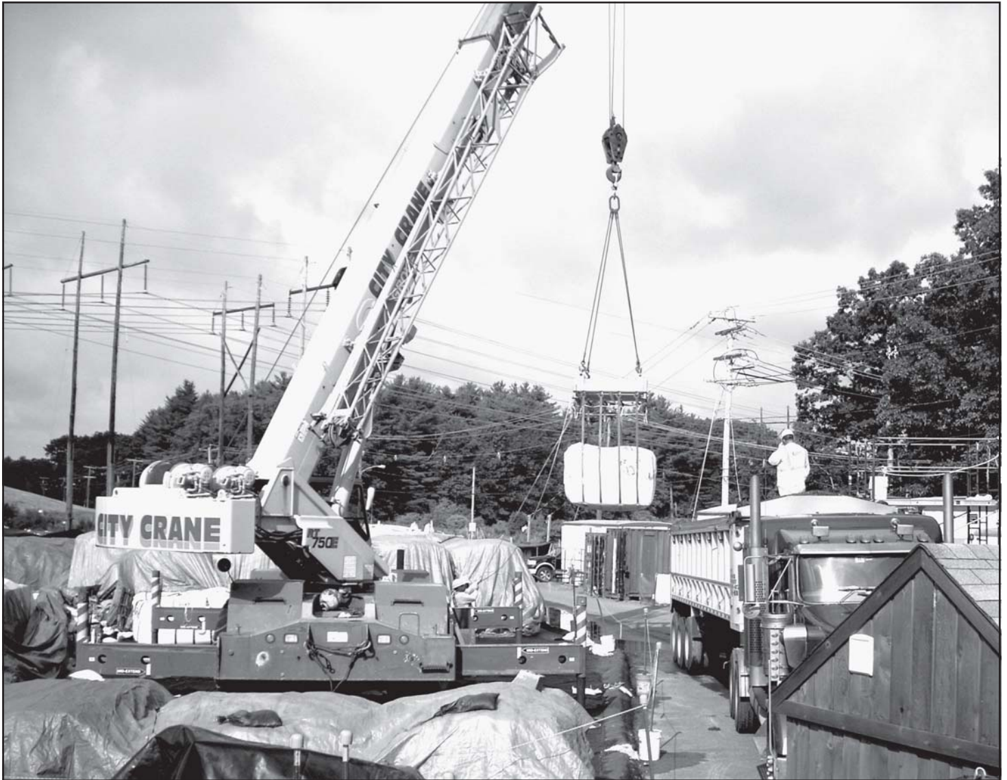
The crane is loading a 10-ton "supersack" filled with contaminated soil into a truck to be shipped off site from the Shpack Landfill for disposal.
