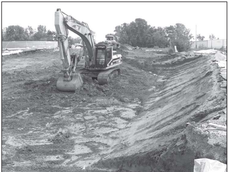
The Corps excavates Survey Unit 10 at the Hazelwood Interim Storage Site property on Latty Avenue at the North County Sites, St. Louis.
