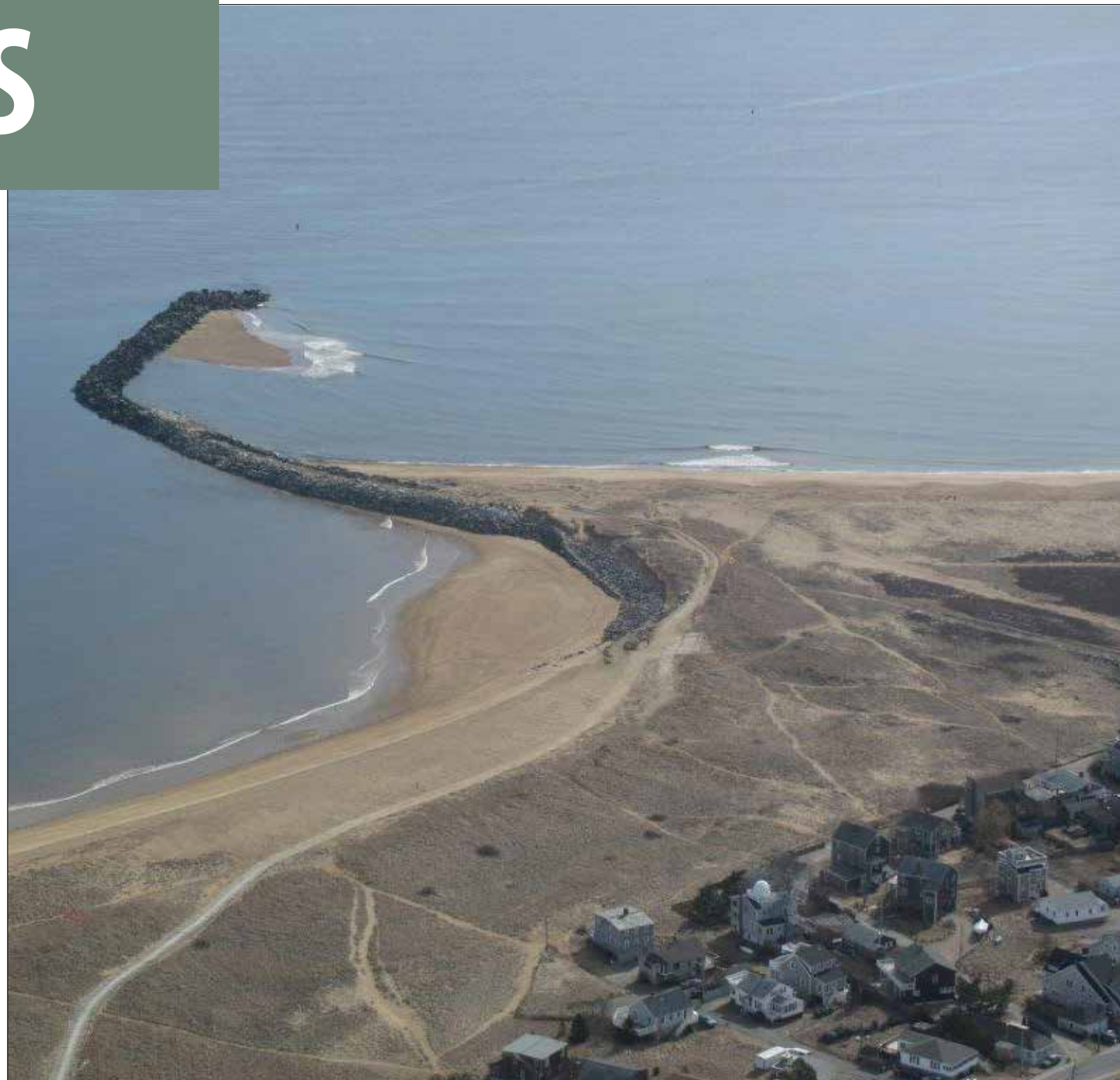
The Newburyport Harbor north jetty in Salisbury, Massachusetts, and the south jetty in Newburyport, damaged during Hurricane Sandy are being repaired by Cashman Equipment Corporation, of Braintree, Massachusetts, under the terms of an $8.2 million contract awarded April 2 by the New England District. Work, which consists of repairing the north jetty in Salisbury and completing repairs to the remaining most seaward 140 feet of the south jetty in Newburyport, is scheduled to take about 12 months to complete. About 30,000 tons of armor stone will be used, including approximately 5,000 tons of 14- to-19-ton armor stone, according to Project Manager Jack Karalius, New England District Programs/Project Management Division. Funding is provided by the Disaster Relief Appropriations Act of 2013. The project will be managed by the New England District. For information on the project visit www.nae.usace.army.mil/Missions/CivilWorks/Navigation/Massachusetts/NewburyportHarbor.aspx . (Courtesy photo)
