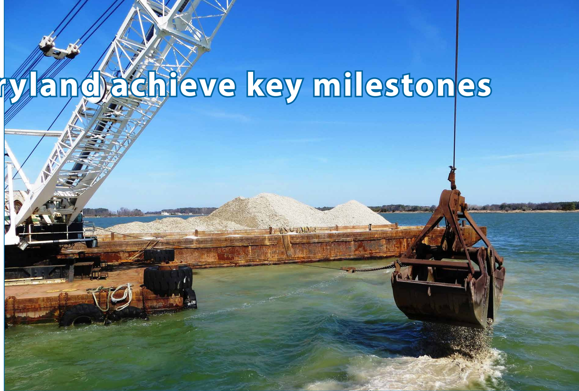
The U.S. Army Corps of Engineers, Baltimore District, places shell to restore oyster reefs in the Chesapeake Bay tributary of Harris Creek April 1. The shell comes from processing plants in the mid-Atlantic region and is permitted to be imported and placed in the river. (Photo by Sean Fritzes)
