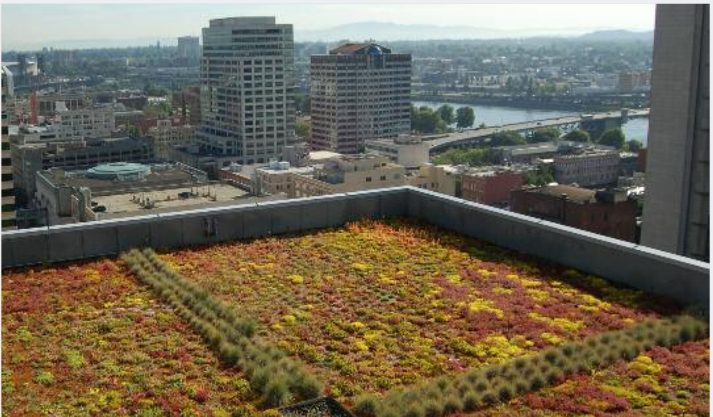
Green roofs in Portland retain 60% of rainfall on average, preventing sewer overflows into the Willamette River.
