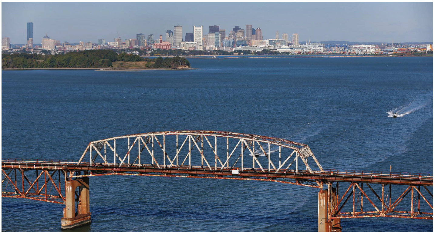
Long Island Bridge located in Boston Harbor in Quincy and Boston, Massachusetts.
