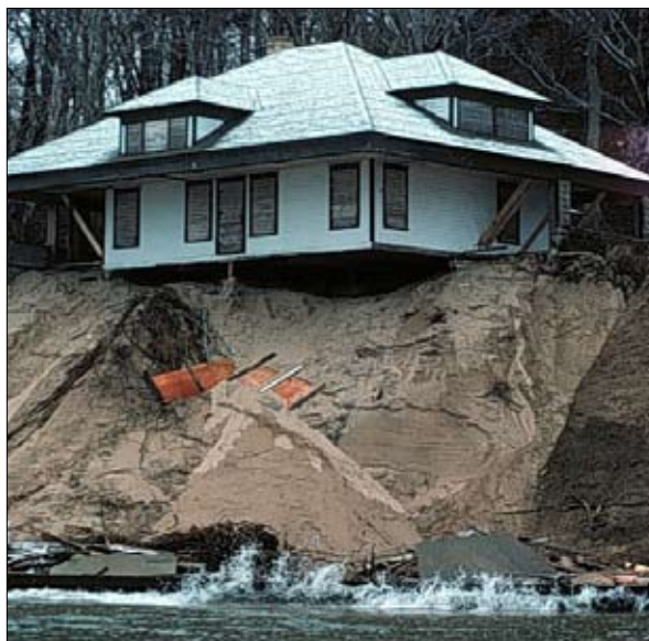
Beach erosion after a storm, Lake Michigan. Source: NOAA GLERL.
