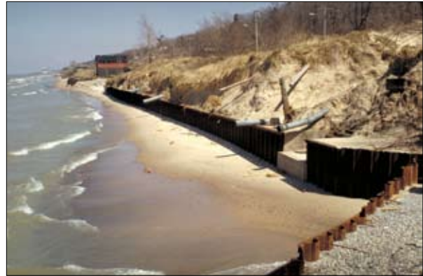
Coastal erosion, Indiana, Lake Michigan. Credit: National Park Service. Source: EPA Great Lakes National Program office.
