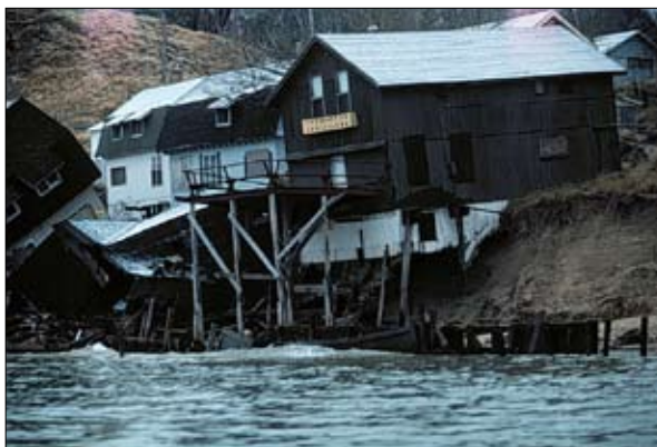
Beach erosion from a winter storm, Lake Michigan. 1985. Source: NOAA GLERL.
