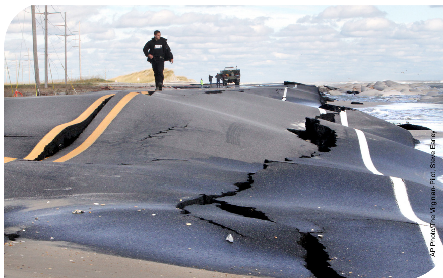
Storm surge on top of rising sea levels have damaged roads and other coastal infrastructure.
