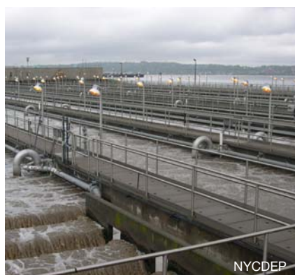
Aeration Tanks at the Hunts Point WPCP
