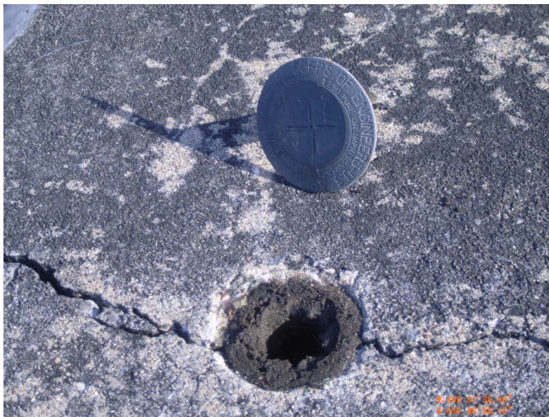
Figure 6-4 Destroyed Monument (irrefutable evidence)
