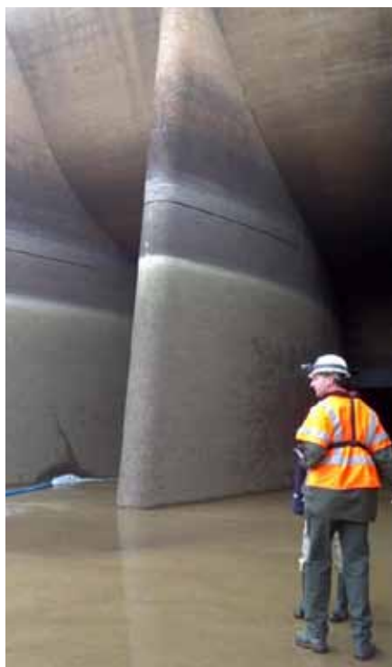
The U.S. Army Corps of Engineers St. Louis District dewatered Wappapello Lake's Dam during the periodic inspection of the Dam and Gatehouse control structure. Photo courtesy of the U.S. Army Corps of Engineers.
