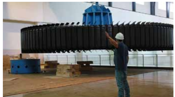
Guiding a 270-ton rotor assembly onto a pedestal at the Barkley Dam Hydropower Plant. U.S. Army Corps of Engineers photo by Lee Roberts.
