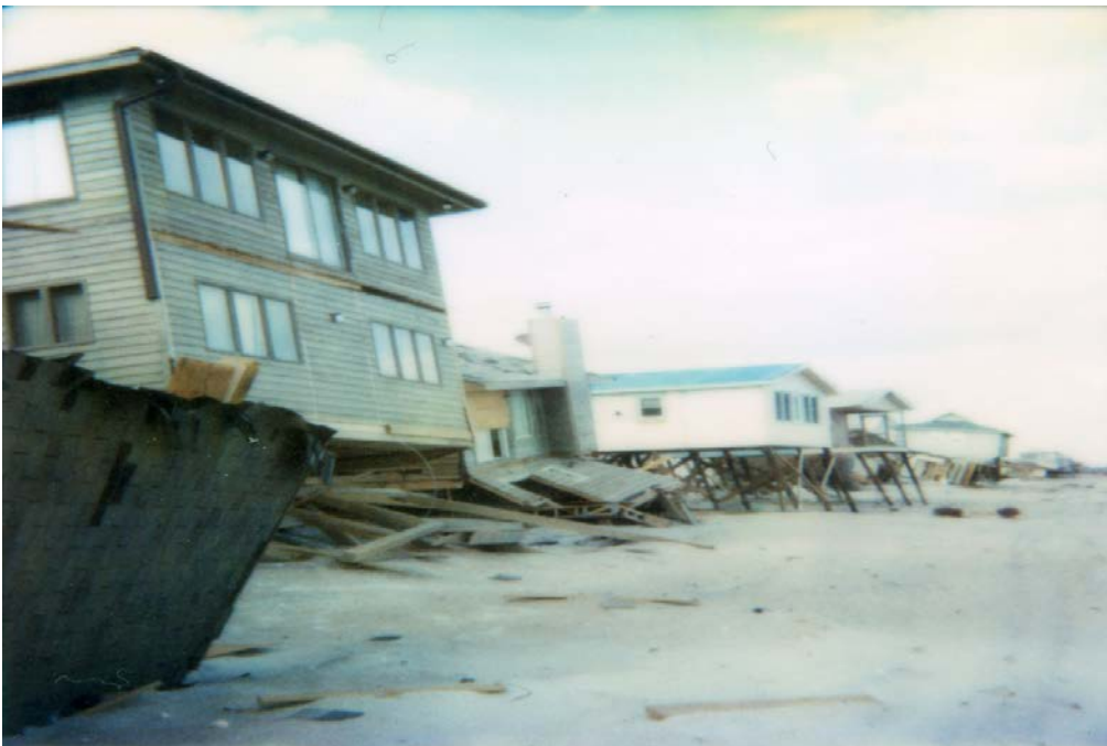
Figure B-4- Coastal storm damage after Hurricane Fran 1996
