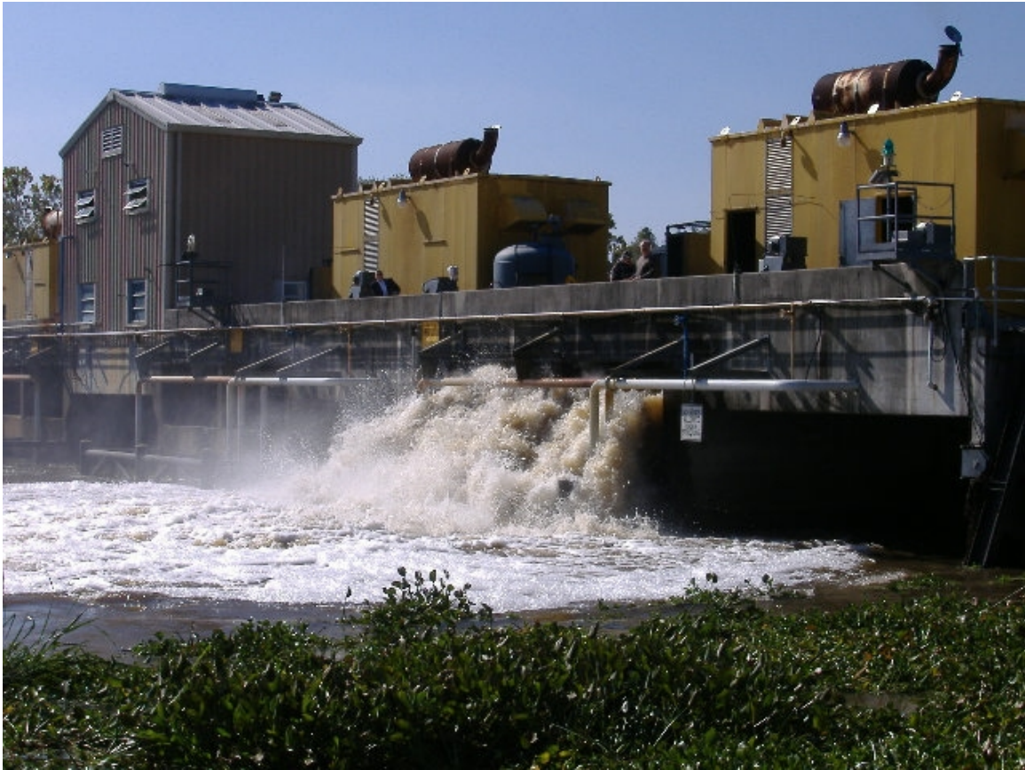
East Ascension Pump Station
