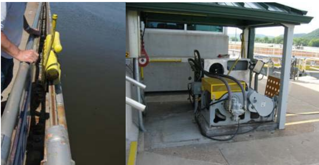
A rail-mounted travelling kevel unit and powered winch system (Photos courtesy St. Paul District)
